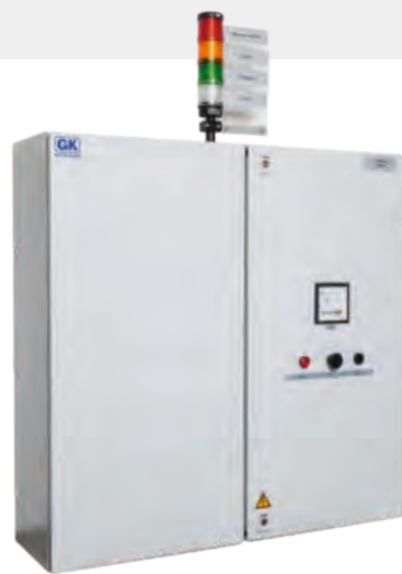
PDU (Power distribution unit)
