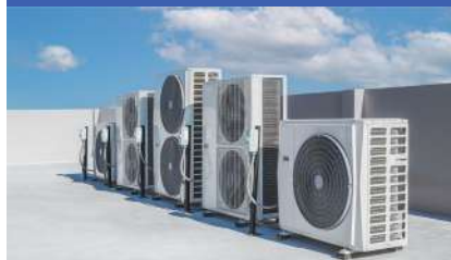
Heat pumps, compressors
